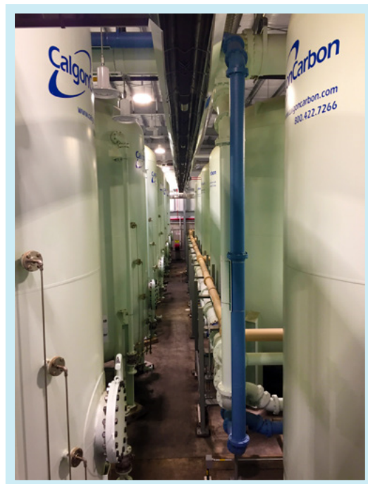
Photo 2: Granulated Activated Carbon filters in Newburgh, used to remove toxic PFAS chemicals from the city’s drinking water. Almost every neighborhood in Newburgh is classified as a PEJA.
