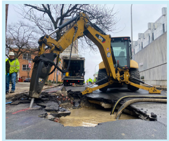
Photo 1: Water main break in Albany.
